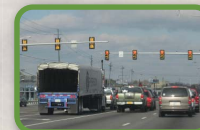
Traffic Signal Coordination System
